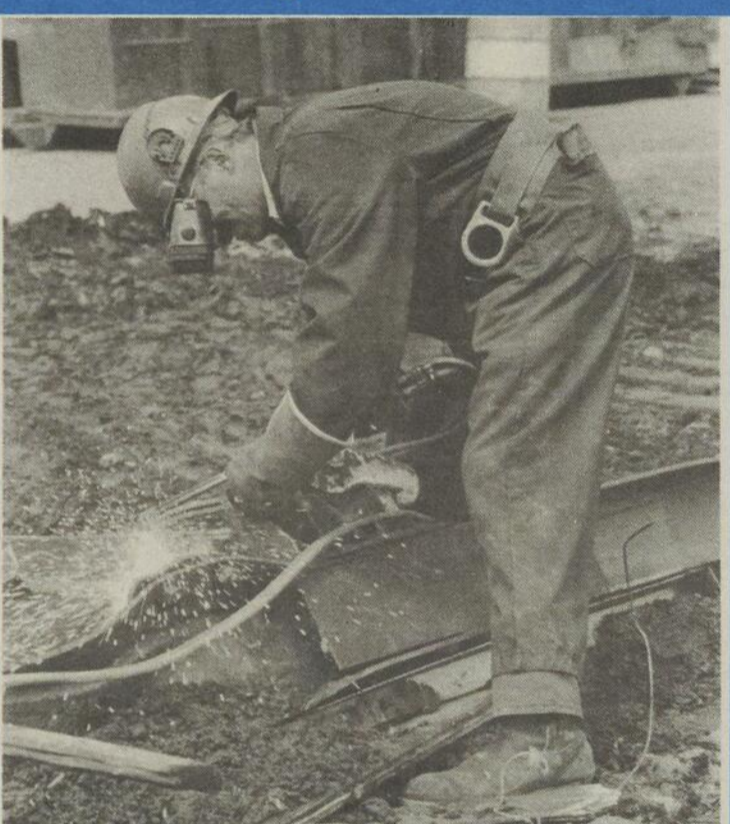
Wrecking crews have spent the last few days tearing down the grandstand at the grounds of the Sherbrooke Fair. For more on the last days of the dilapidated former showplace, please turn to Page 4. RECORD: GRANT SIMEON
