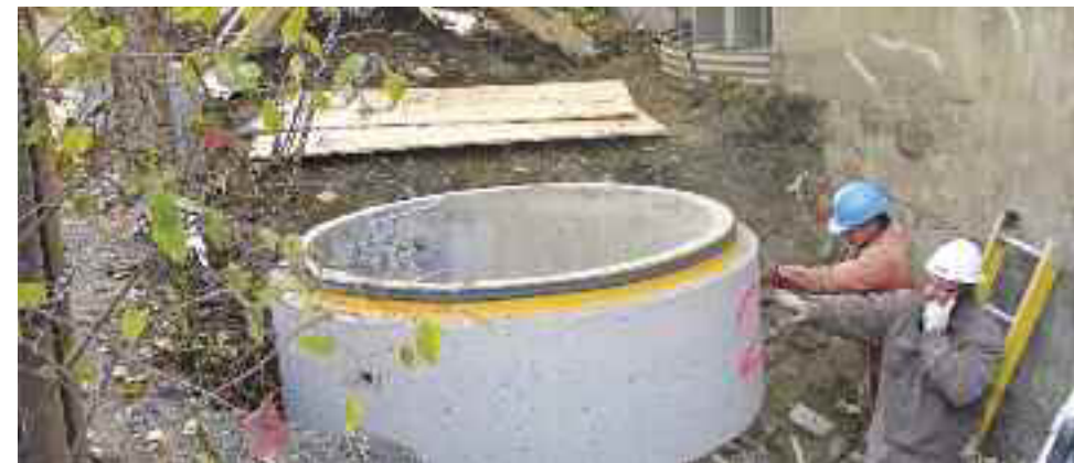
At the southeast side of Westmount Park Church, workers lower a concrete section of an access chamber to an old manhole November 8 as part of a project to cap a century-old pipe draining into the site of the Westmount recreation centre.
