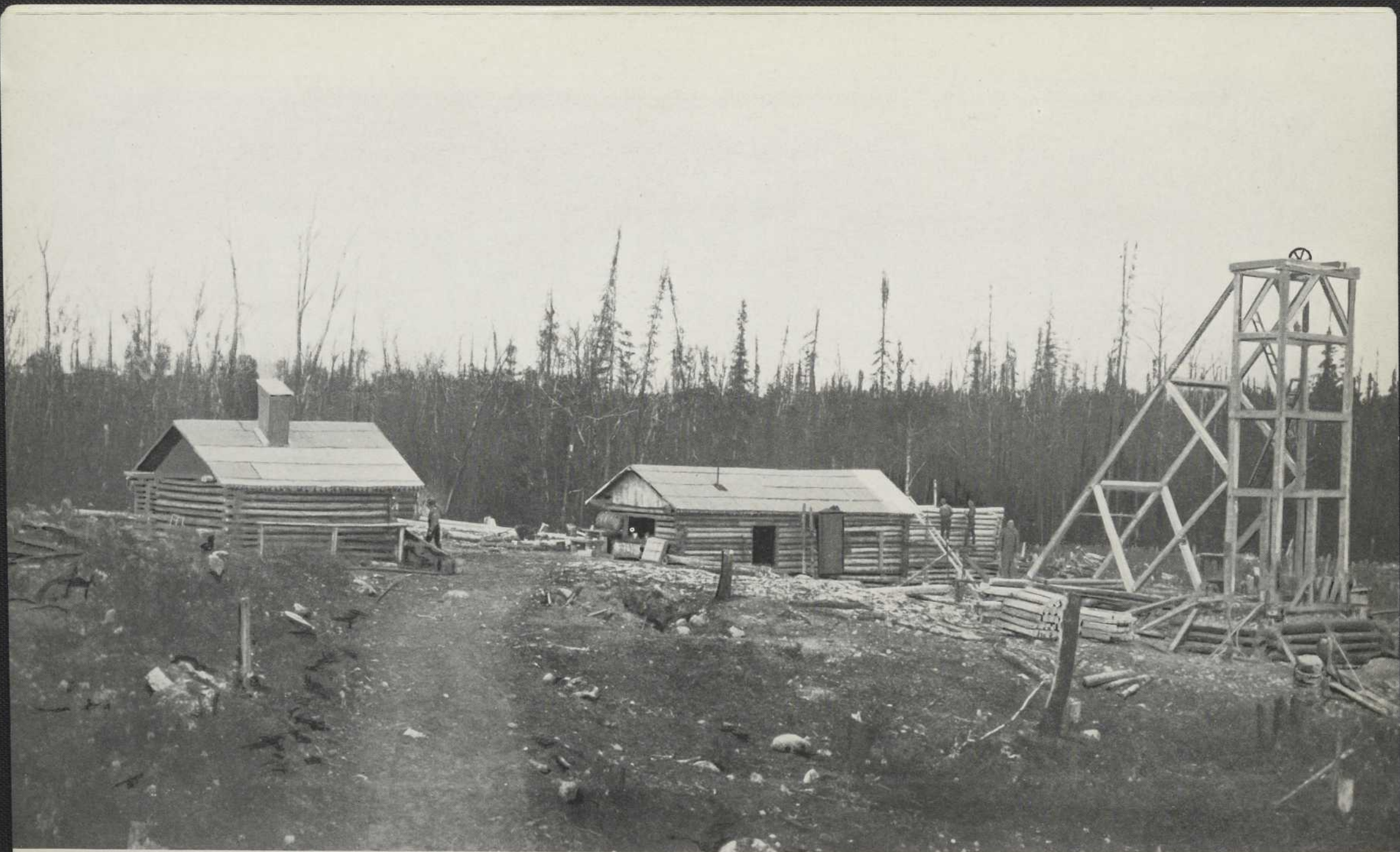
51 THEN Aldermac Mines, Limited (Beauchastel township, Témiscamingue county). Erecting the first camps and machine shop in 1928.
