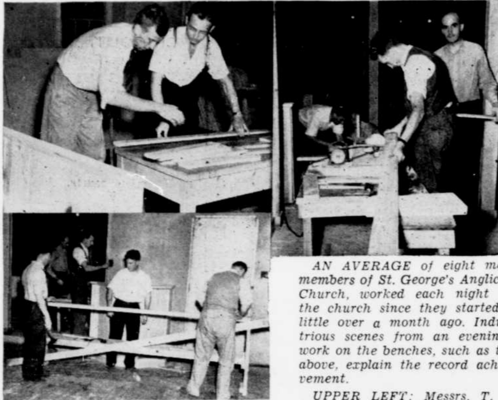
AN AVERAGE of eight men, members of St. George's Anglican Church, worked each night on the church since they started a little over a month ago. Industrious scenes from an evening's work on the benches, such as the above, explain the record achievement. UPPER LEFT: Messrs. T. L. Brock and Merle Washburn finish off a completed bench; LOWER LEFT: (front) Messrs. Karl Stewart, Ben Young and G. Craig assemble a frame. UPPER RIGHT: Messrs. G. Gale and J. Collins cut pieces for back of bench. Mr. Young and Mr. Stewart are seen in background.
