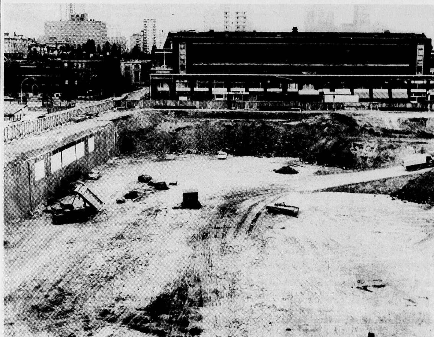
THAT'S A HOLE? This is the hole that has been dug for the West-End Plaza. It has to be the biggest hole ever dug in Westmount. It measures the best part of a full city block in area and it will house a multi-level garage. See Page 4.
