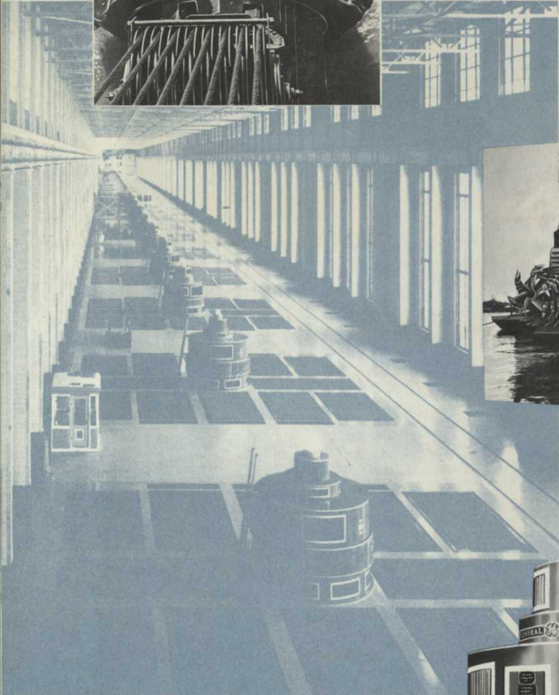
Interior view of the Beauharnois Power House. The 2,200-foot building houses 14 generators of 40,000 kilowatts, 53,000 horsepower capacity apiece, and 12 units of 41,000 kilowatts, 55,000 horsepower capacity apiece.
