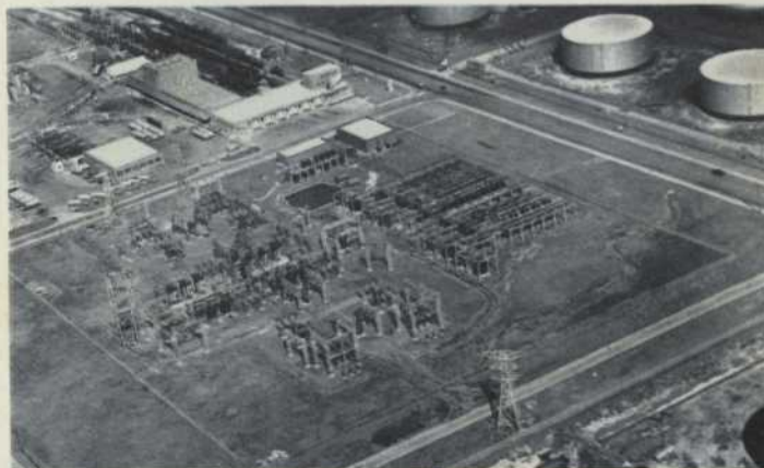
Montreal East Stn. 135,000 KVA — 120/12/4KV
