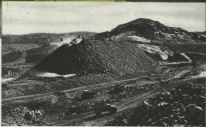
The main dam on the Bersimis River is 2,210 feet long, 200 feet high and 900 feet wide at the base, with a 40-foot wide crest.
