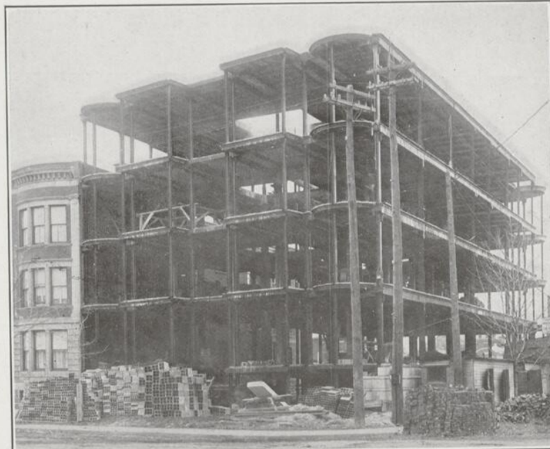
EXTRAORDINARY BUILDING DEVELOPMENT IN MONTREAL EXTENDS TO WESTMOUNT—View of the new Western Apartments situated at the southeast corner of Western and Oliver avenues. This building will be one of the most palatial apartment houses on the island of Montreal, and is especially the last word in fireproof construction. It will be ready for occupancy by Sept. 1st next. It is being built by the Montreal Construction Company.
