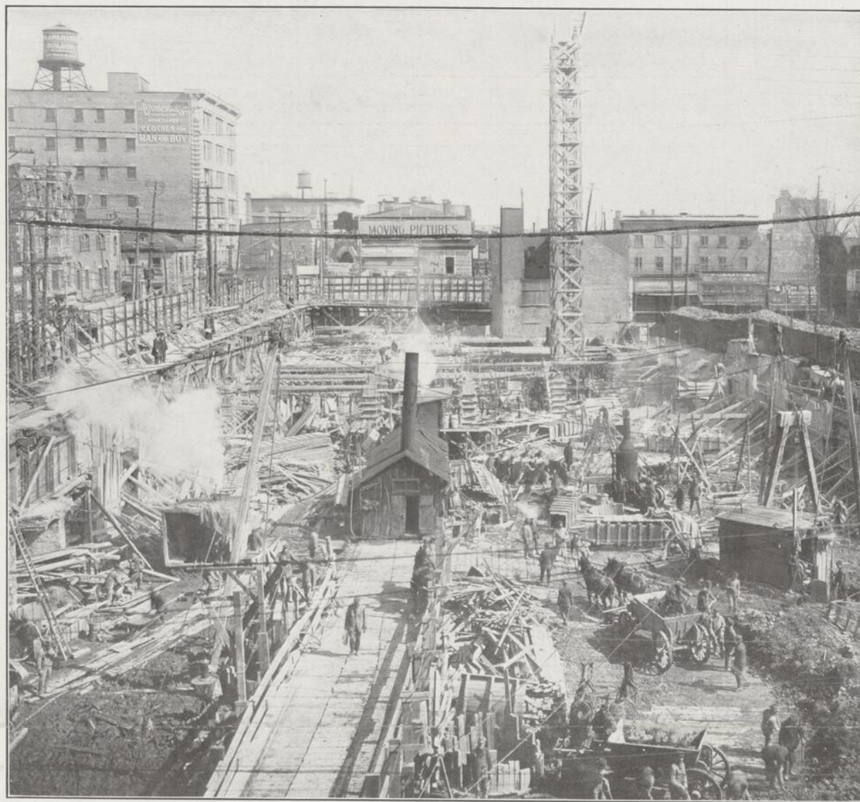
MODERN MONTREAL—Digging the heart out of St. Catherine street. A unique and wonderful picture of the operations now going on in the building of the immense new Scroggie Departmental Store which will occupy the whole block between Bleury, St. Catherine, Alexander and St. Edward streets. Work on this building has been going on apace and the building is expected to be completed next autumn. By this enormous building, St. Catherine street at this point will be immensely improved.
