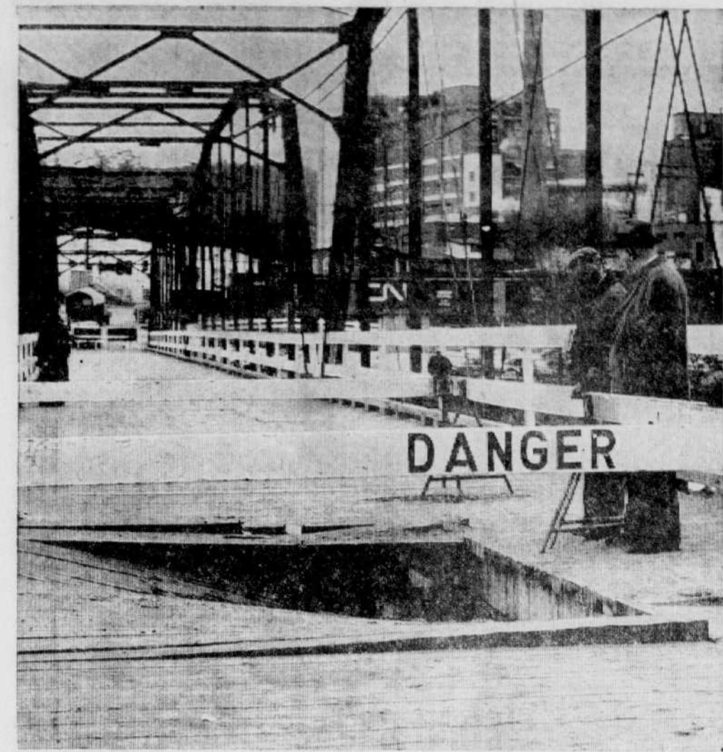
WRECKED BRIDGE — Harold Robinson, left, a Greenlay truck operator, and a Sherbrooke Record reporter, examine the damage caused to the Windsor-Greenlay bridge when a heavy truck went through the 60-year-old structure Monday morning. Provincial Public Works Department officials are expected to start repair work late today or Wednesday morning. (Record Photo by Gerry Lemay)
