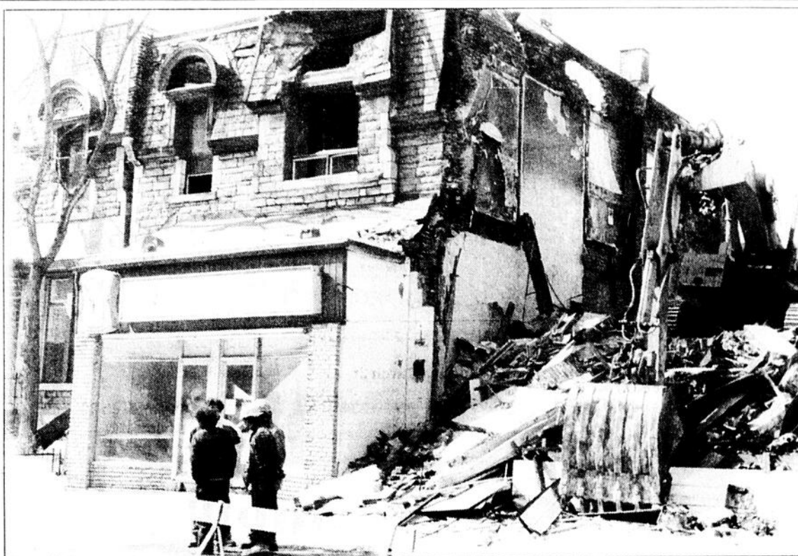
Demolition crews struck a gas pipe Wednesday last week at the site of the former Westmount Bar B Q building at 4469 St. Catherine St., destroyed in an arson fire Nov. 28.
