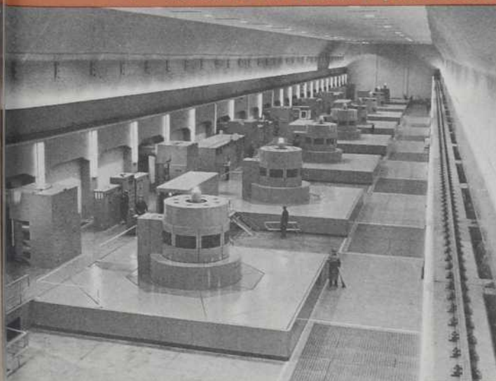
▼ Interior of the Bersimis I power-station.
