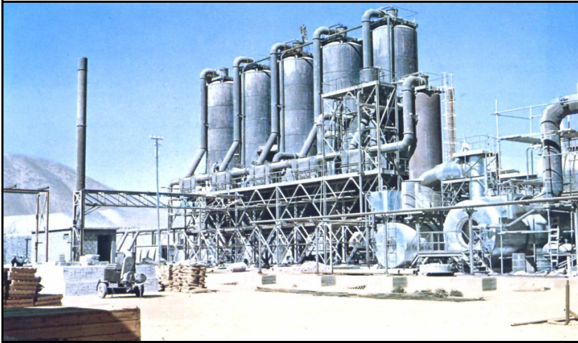
Figure 1.98: Sulfur dioxide towers for precipitating \text{Cu}_2\text{Cl}_2 .
