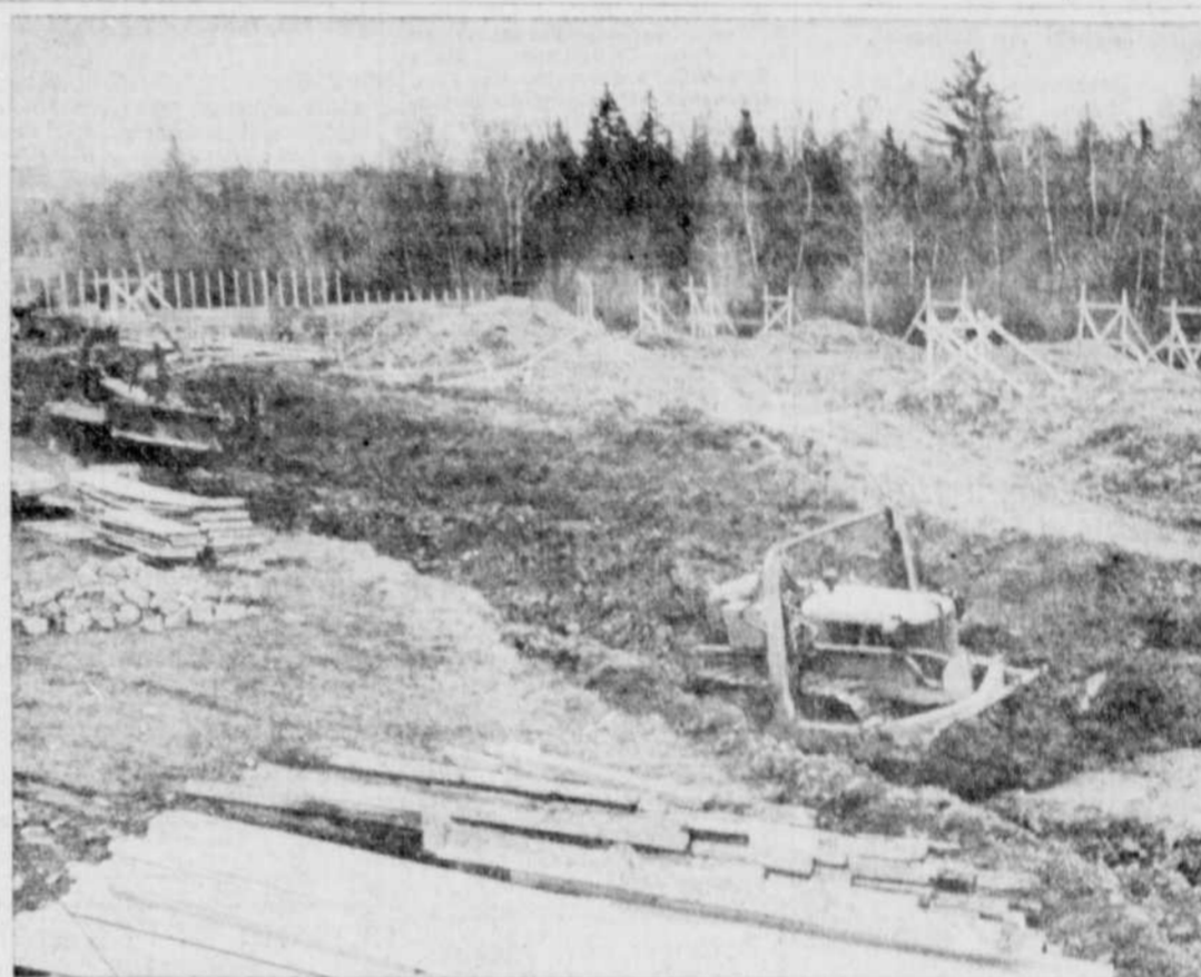
EXCAVATION STARTS — Work of excavating for the new women's residence at Bishop's University was started during the past week. (Record photo by Gerry Lemay.)
