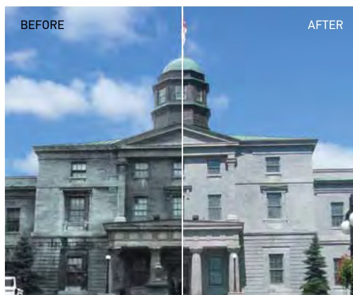
The cleaning and restoration of the masonry on the iconic, 169-year-old Arts Building reversed many years of weathering and deterioration on a building that is so symbolic of McGill's deep roots and traditions.
