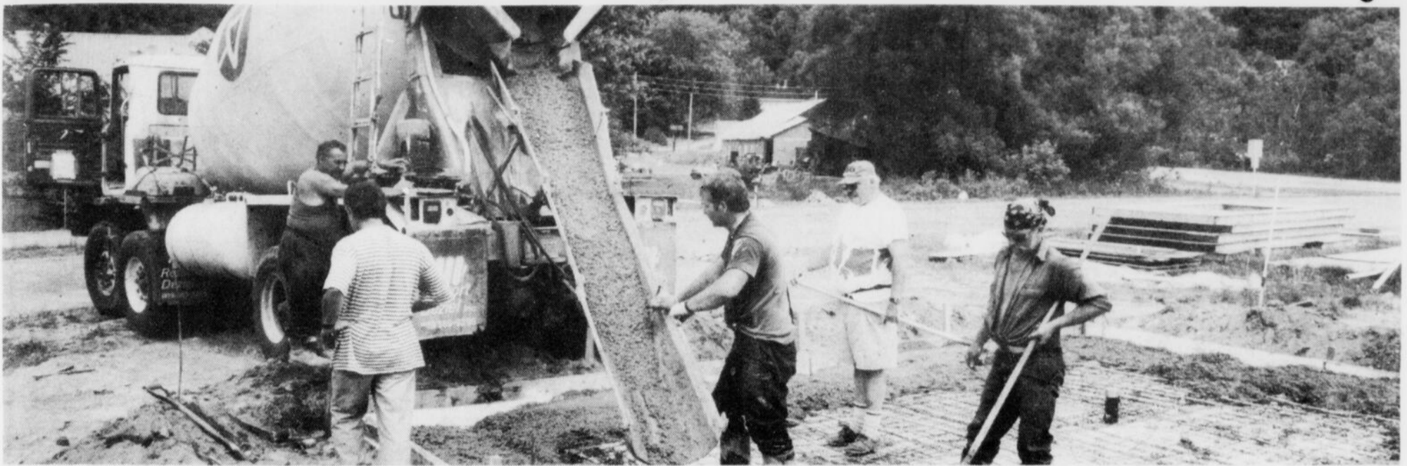
Yvan Dagenais, Ron Smith and Richard Cliche of Vision 2000 take receipt of a load of cement last summer, used in the floor of the new changing rooms.
