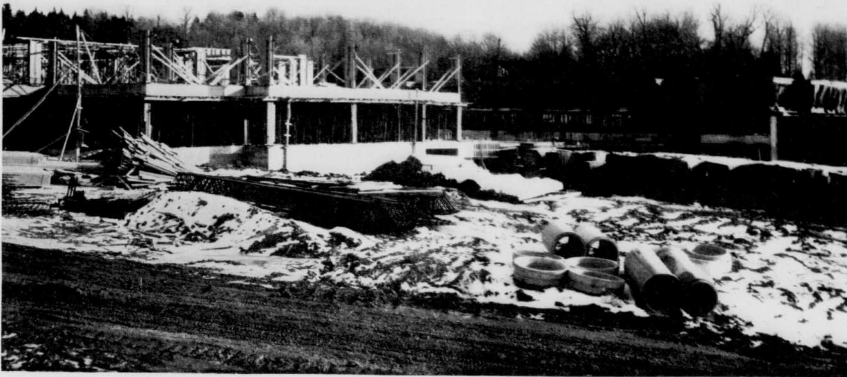
GOING UP — The 260 men working on the construction of the ET Regional High School are working long hours to finish the school for September 1, 1969. Yesterday, large trucks rolled through the muddy paths, men hammered and sawed and the buildings seemed to grow every hour. The school gymnasium, not seen in the picture, is nearly completed. The school is located near Lennoxville. (Record photo: Gerry Lemay)
