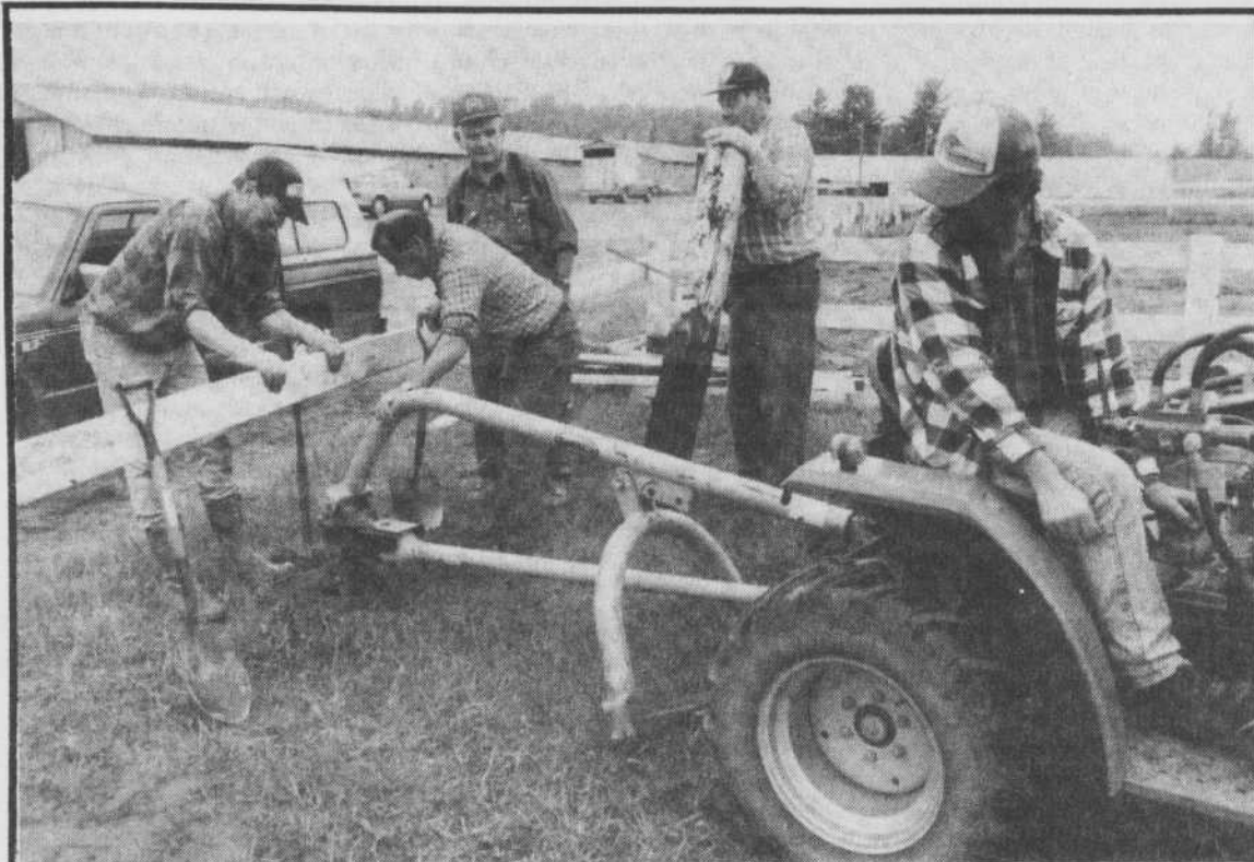
Finishing touches: Peter McHarg, Arnel Grenier, Richey Harrison, Marvin Smith and Len Young were putting in some of the last posts in the new board fencing on the Ayer's Cliff fair grounds Sunday, the last in a series of renovations to the fairgrounds. Now the grounds will be spruced up for the monthly horse shows and the fair in the late summer.
