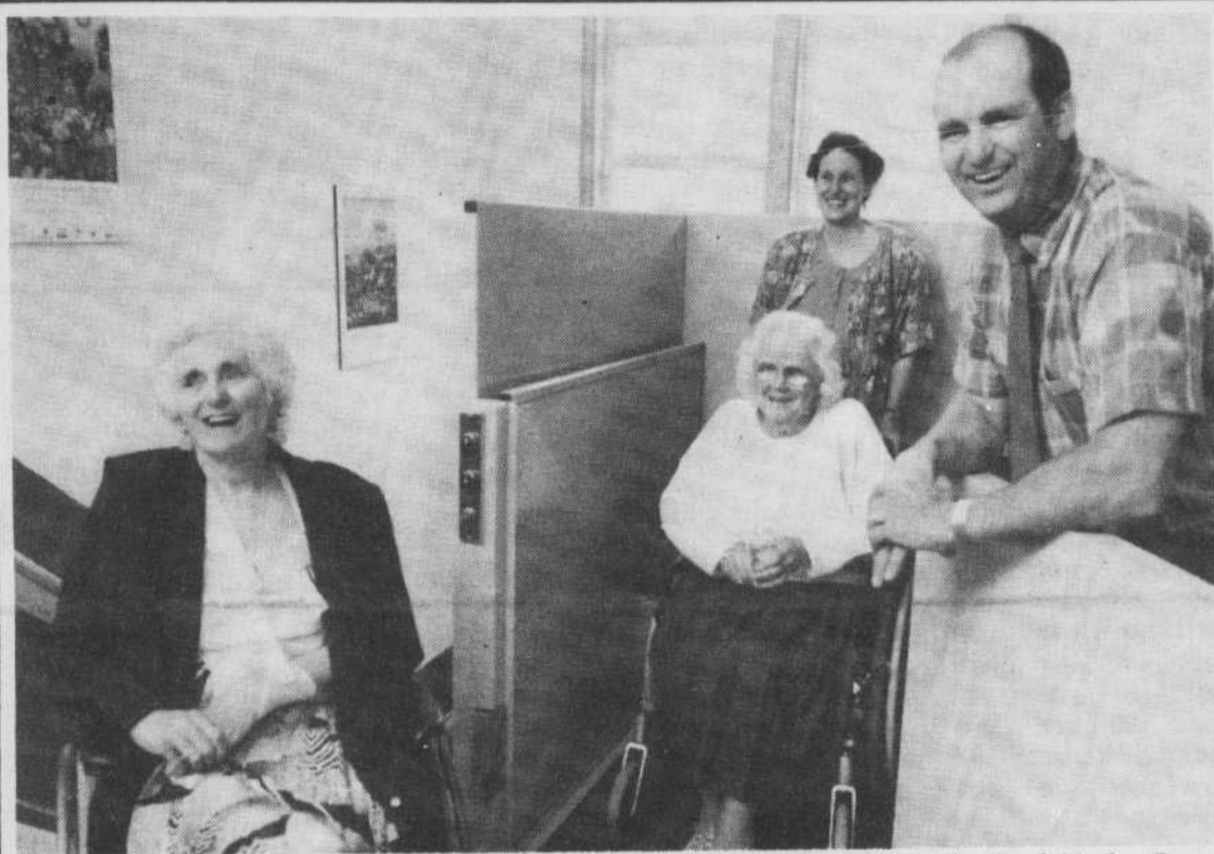
Imogene Browning and Kay Gallop will now have an easier time getting into the North Hatley Community Centre thanks to the installation of this new lift. For more on the story, see inside.
