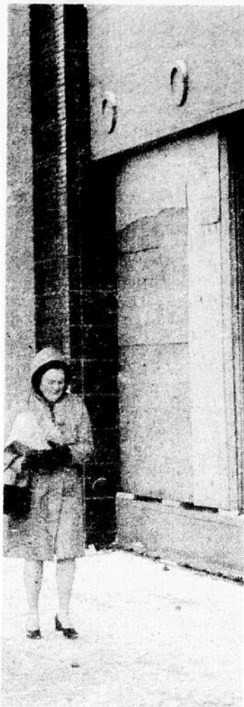
STORM VICTIM: This Sherbrooke street window of the Steinberg's store at Victoria avenue was a victim of Monday's high winds. The store was forced to close before boards could be put up and warmth restored inside.
