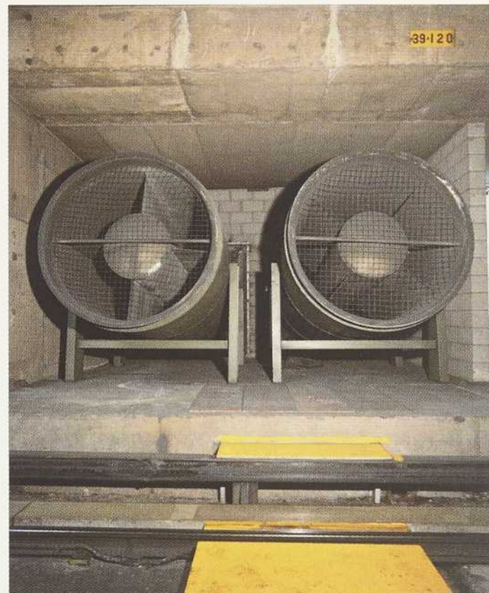
Ventilation units inside tunnel. (STM Archives)
