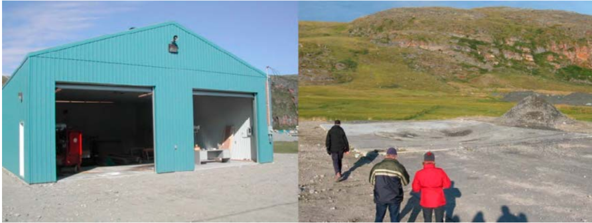
FIGURE 5.49: SALLUIT FIREFIGHTERS' GARAGE. BUILT IN 2003 ON A CONCRETE SLAB, IT HAD TO BE DEMOLISHED AFTER THE FLOOR SANK ABOUT 0.50 M DUE TO THAWING OF THE PERMAFROST UNDER THE FOUNDATION.
