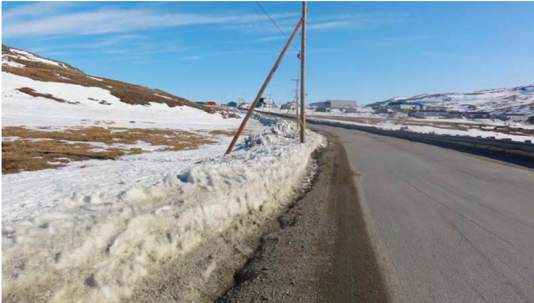
FIGURE 5.48: LARGE ACCUMULATION OF SNOW AGAINST FILL ON THE AIRPORT ROAD AT SALLUIT IN MAY 2011. THE ROAD HAD TO BE REBUILT IN 2012 TO REPAIR THE DAMAGE CAUSED BY PERMAFROST DETERIORATION.
