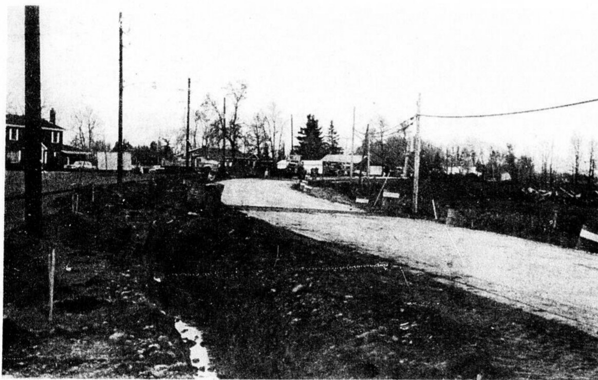
As photo shows, deep ditches have been excavated on both sides of Route 138, just out of Huntingdon. It's not known when the work will be completed.
