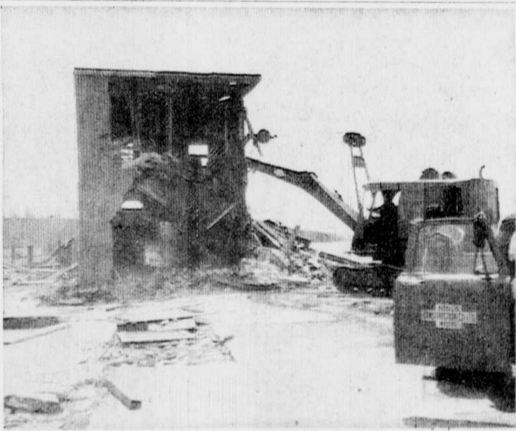
BUILDING PARK AT MAGOG — The wreckers moved into Magog last week when remains of the former MacPherson mill were demolished prior to operations that will turn the lakeside site into a recreational park and beach area.
