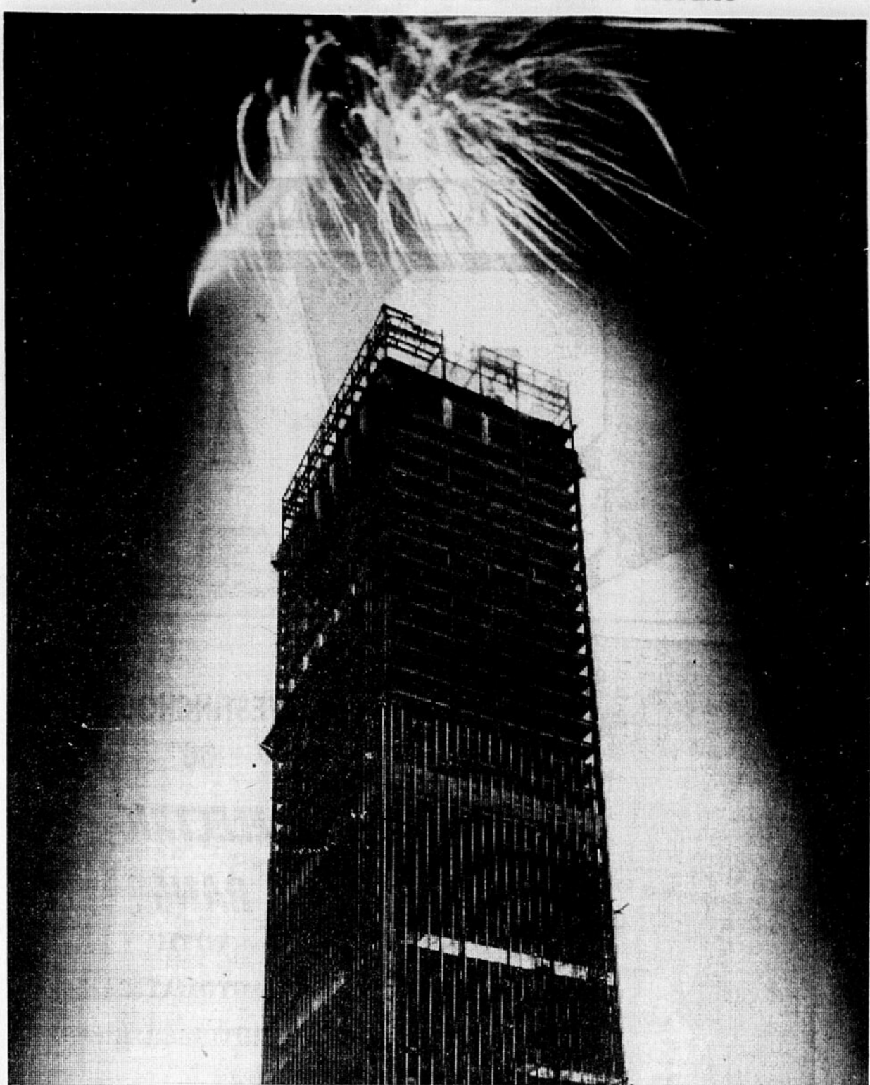
Brilliant fireworks against low rain clouds lit the Montreal sky as the last girder was swung into position atop the 604 ft. Canadian Imperial Bank of Commerce building, tallest in the Commonwealth. The gilt-painted 18-ton girder was illuminated by search lights as it made its ascent.
