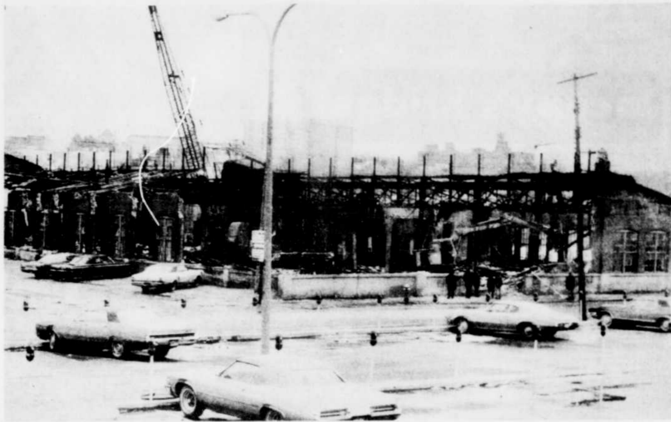
WHAT GOES UP... — Workmen had the task of demolishing the former James United Steel building on Grandes Fourches Street in Sherbrooke. Speculation continues as to the ultimate
