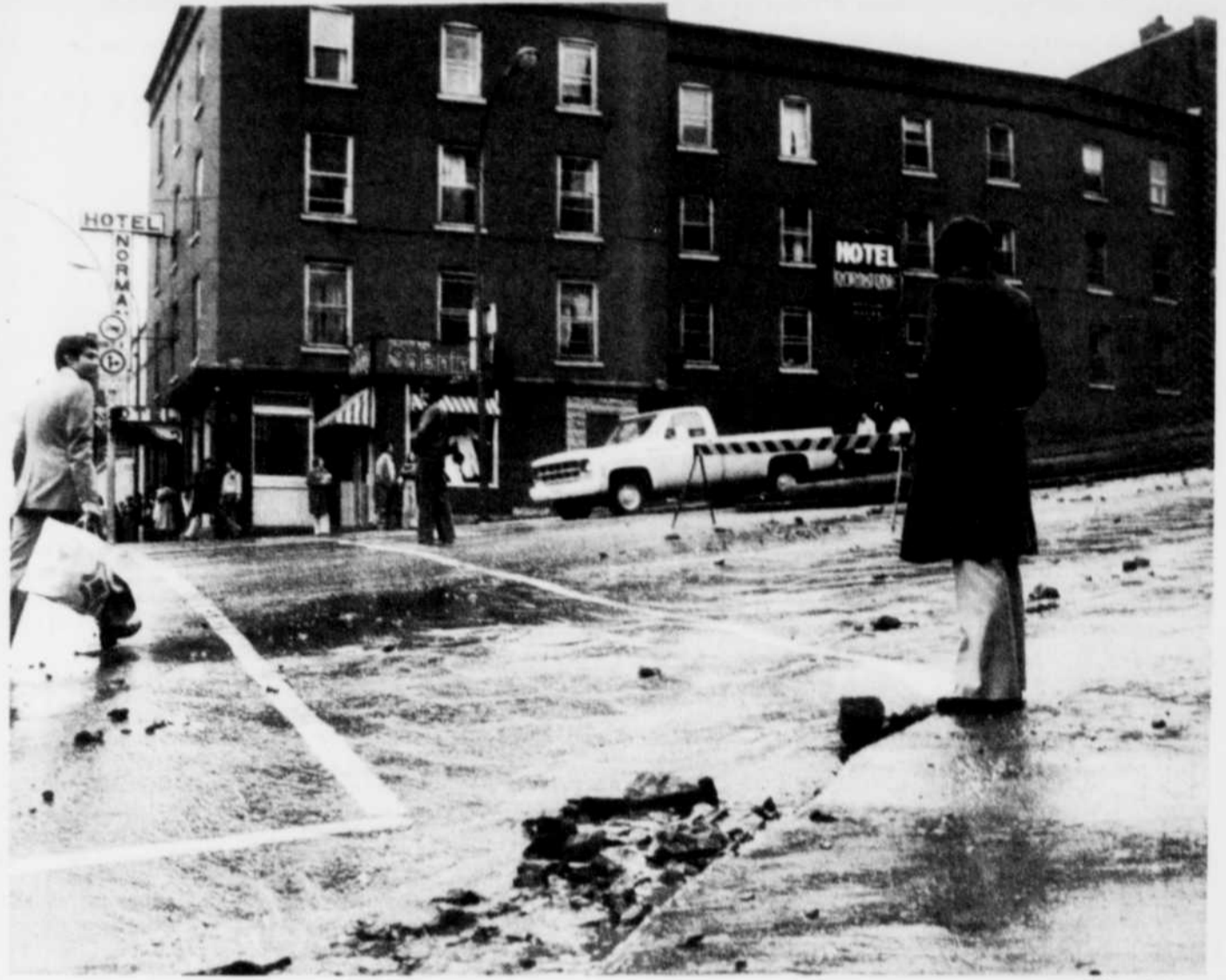
The old Normandie will be coming down during the wee hours of Saturday, its demolition contractor assured the city last night.
