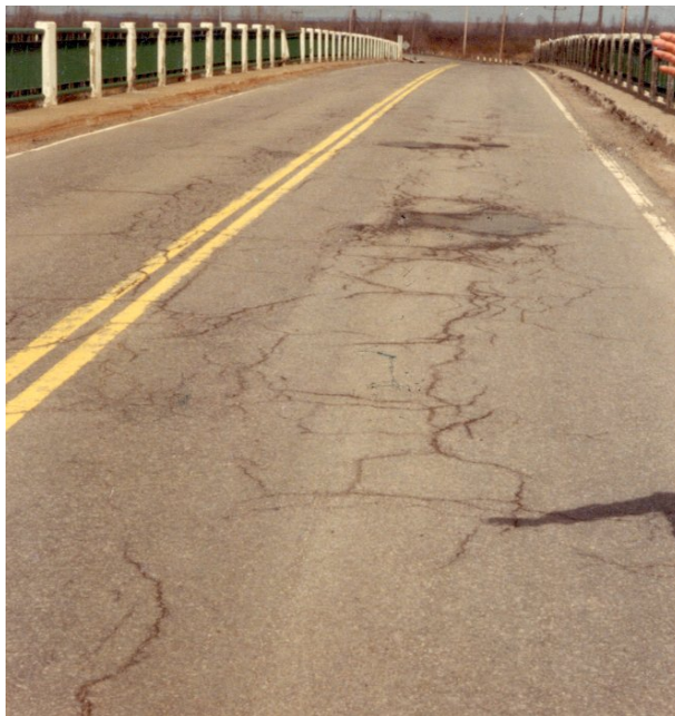
Photo 4.7-1 c) – Fissures polygonales
