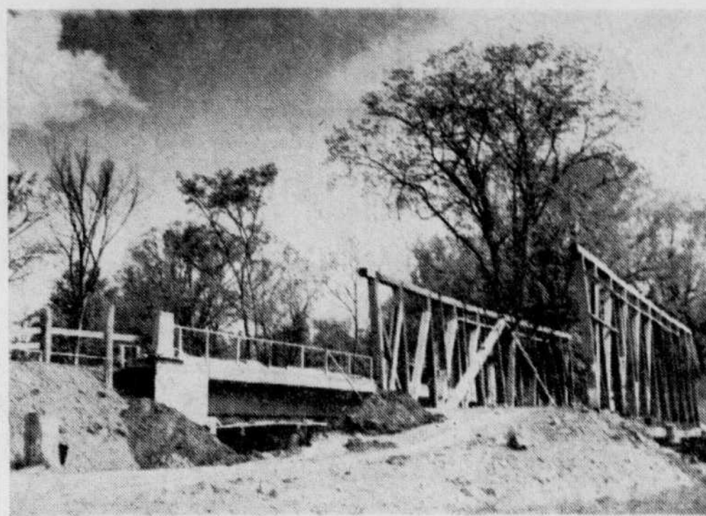
SKELETON IS ALL THAT REMAINS — The side and roof of an old covered bridge, right, over the Coaticook River on the Hatley Road within the municipal limits of Compton, have been removed. At right is the bridge recently
