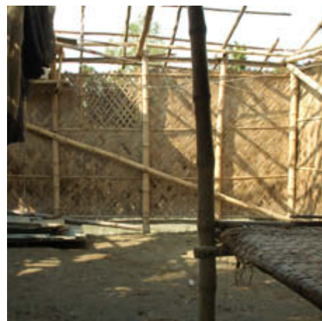
Interior (roof damaged by cyclone)
