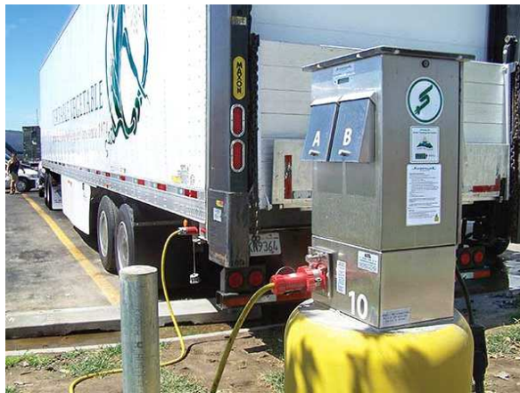
(a) Electrified Parking Space
