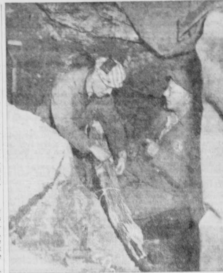
WHICH IS WHICH? — Bell Telephone employees Euclide Lalonde and J. C. Barron of Coaticook repair a cable containing 1,200 wires in Stanstead. The cable was damaged during excavation operations for the Sunnyside School addition, disrupting service temporarily. (Record Photo by Pepin)
