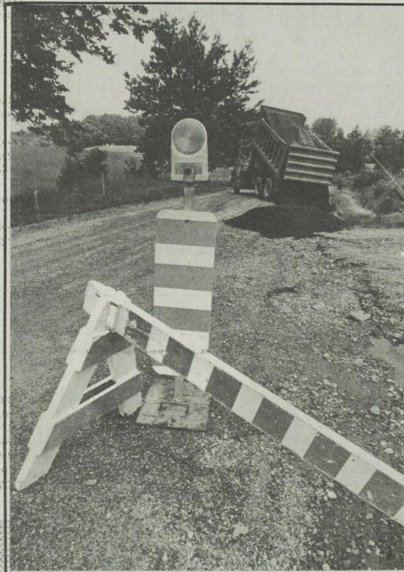
Fixing the damage: Workers were out on the Ascot roads after the storm Saturday washed away more than one shoulder. On Bartlett Road (above) the shoulder fell by almost six inches in the heavy rains. Crews will be out again coping with problems caused by the weather.
