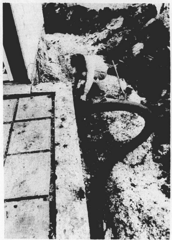
David Smith installs a drain pipe with a filter against glass dust.
