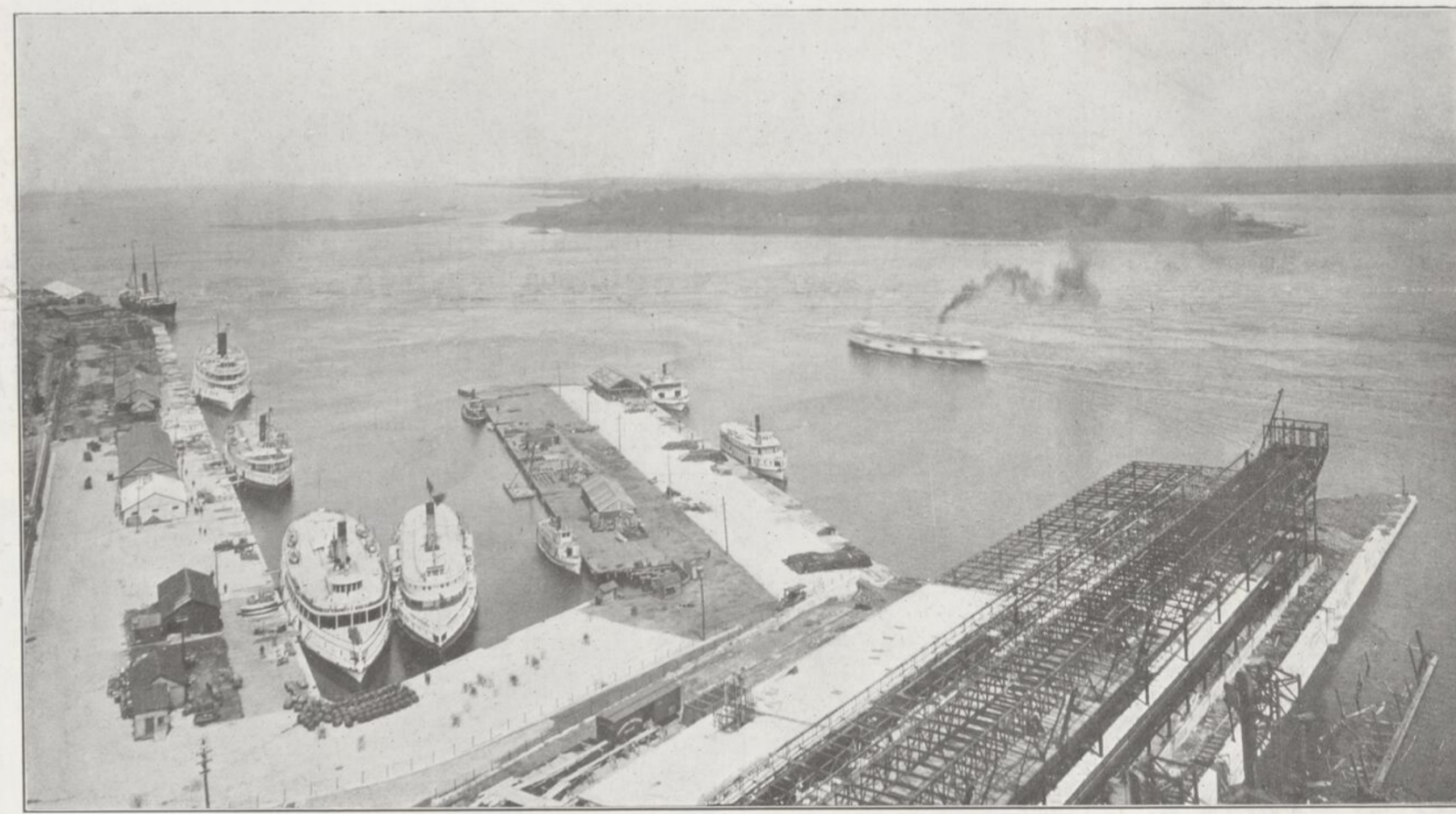
NEW AND STRIKING VIEWS OF MONTREAL —The eastern portion of the harbor front as seen from the Harbor Commissioners' Elevator No. 2. In the foreground one of the 14 new steel sheds may be seen in course of construction. Beyond is the low-level Victoria Pier, at which many British and foreign men-of-war have been warped during the past three decades. In the background is St. Helen's Island, once the property of Samuel de Champlain (the name of whose wife it bears), founder of Quebec and discoverer of the Great Lakes. To this Island the Marquis de Levis, commanding the last French Army, retired in 1760, and there burnt his flags in the presence of his army on the night previous to Vaudreuil's surrender of the Colony to General Amherst.
