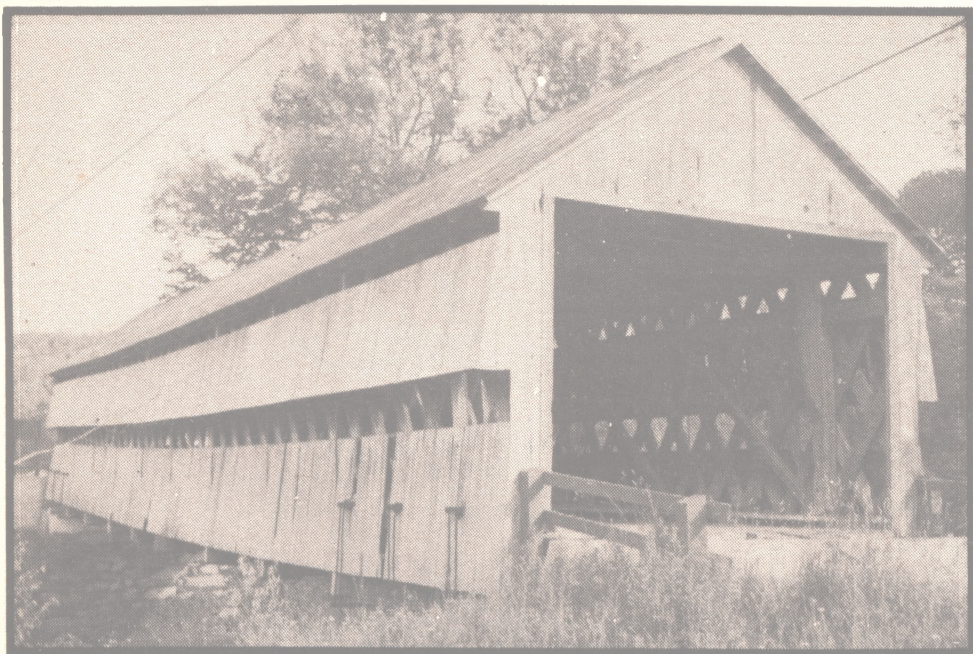
Despite the heavy sag in the Capelton Bridge, the "town" style lattice structure remains strong. As discovered in Vermont the only way to remove it is piece by piece—a wrecking ball is useless.
