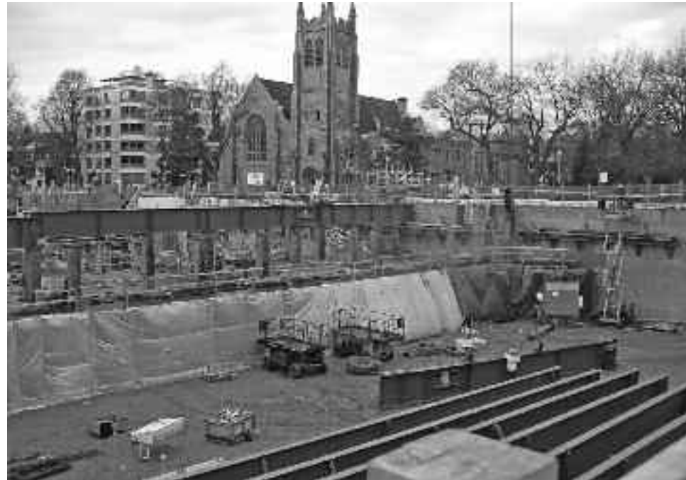
The east rink December 4 just before steel roof beams (in the foreground) were lifted into place.
