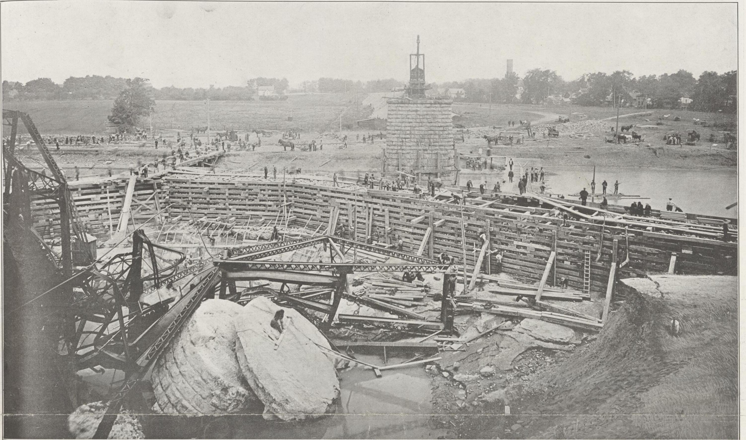
REPAIRING THE HUGE BREAK IN THE EMBANKMENT OF THE CORNWALL CANAL—The above illustration shows the huge crib that had to be built and filled in before the task of dredging a new channel could be proceeded with. The old embankment, as well as the pivot pier and ruins of the railway swing bridge, may be seen in the foreground. By dint of almost superhuman exertion, the big break was repaired in less than three weeks' time—a notable achievement.
