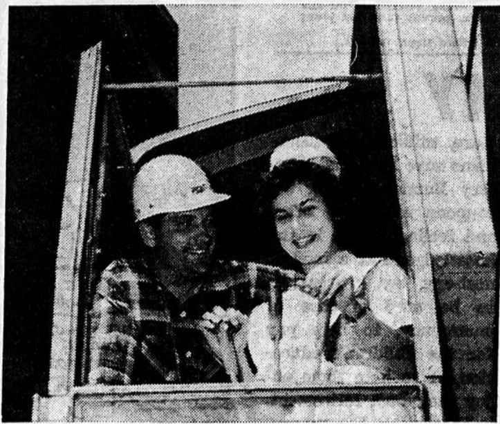
FROM NURSING to operating a steam shovel was all part of the line of duty for young Ruth Lennox as she turned the sod for the extension of the Queen Elizabeth Hospital and accompanied job superintendent Frank McCormack on the big power steam shovel that is taking over the job. Miss Lennox is the hospital's youngest nurse.
