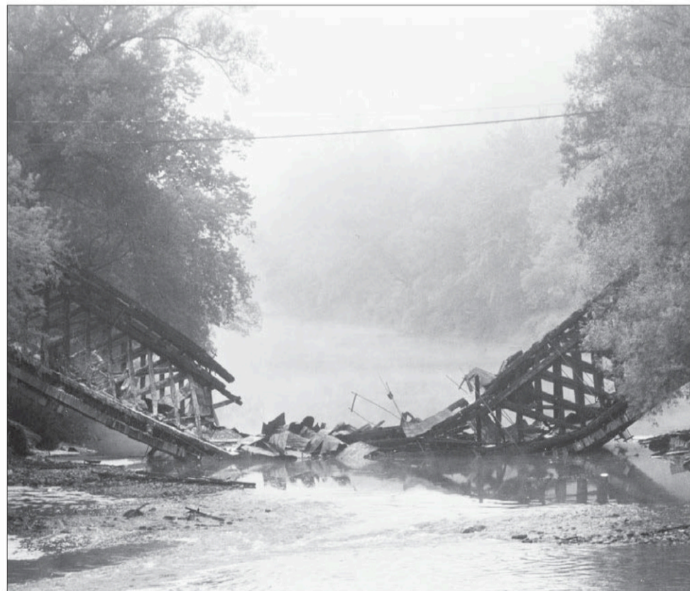
The Capelton bridge on the morning of September 18, 2002, after being razed by fire. Photograph by Michael Grayson (P235 Michael Grayson fonds)
