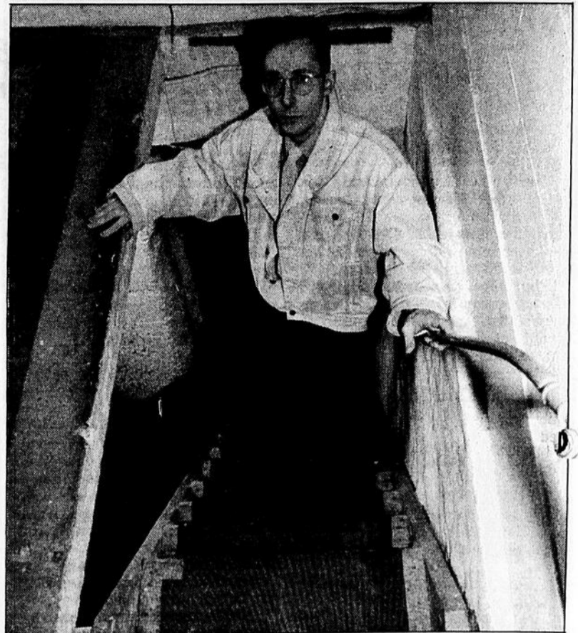
Gilles Gardner stands on narrow steep steps leading to the laundry room at 4123 de Maisonneuve. Notice there is no outside guard rail.
