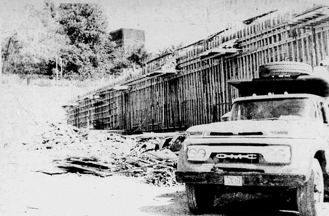
NEW HYDRO SUB-STATION: Once the subject of bitter dispute, when first announced to be located in the Clondeboye-Prospect area, the new sub-station for Quebec-Hydro is now rapidly taking shape in what had been Selby Park. Top view shows the structure's west side—that's the top of Westmount Square over the top of the hill. The lower view, taken from south of St. Antoine street, shows the east side of the massive concrete building this week.
