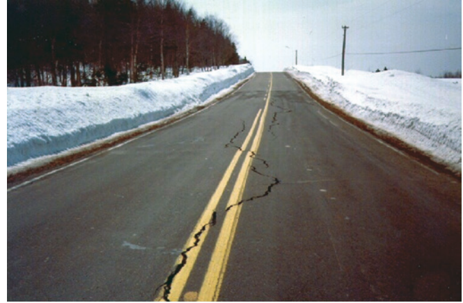
Longitudinal cracking, as depicted in Figure 2
