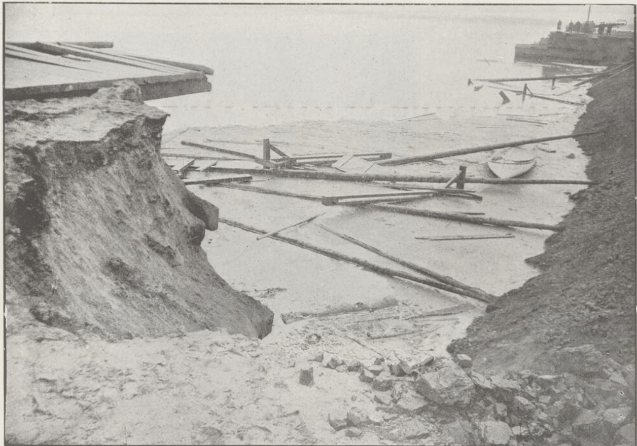
THE DAMAGED WHARF AT SOREL, QUE.
