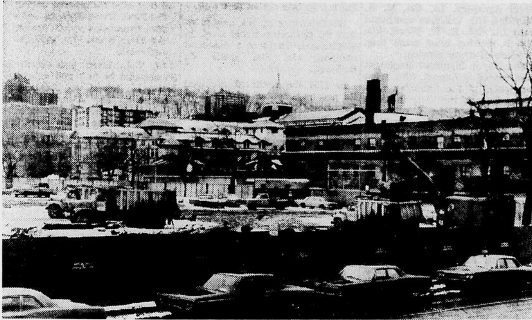
UNDERWAY: Digging begins on the site of the Westmount Square complex, a $25,000,000 project being built by the MonDev Corp. in the
