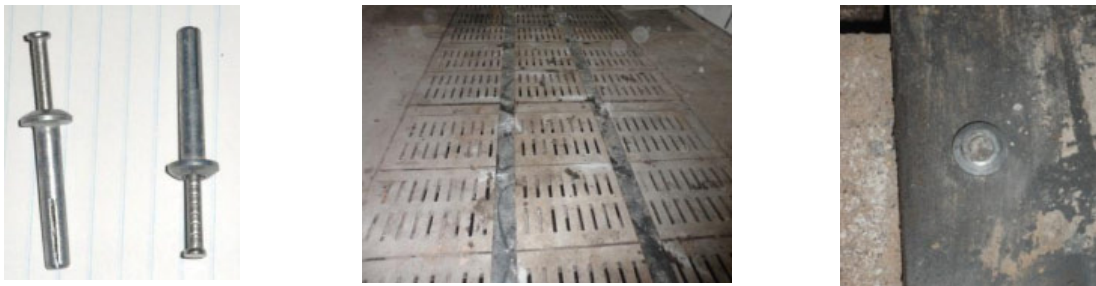
Figure 15 Use of stainless steel rivets and long metal plates to seal the manure slides of the gestation slats
