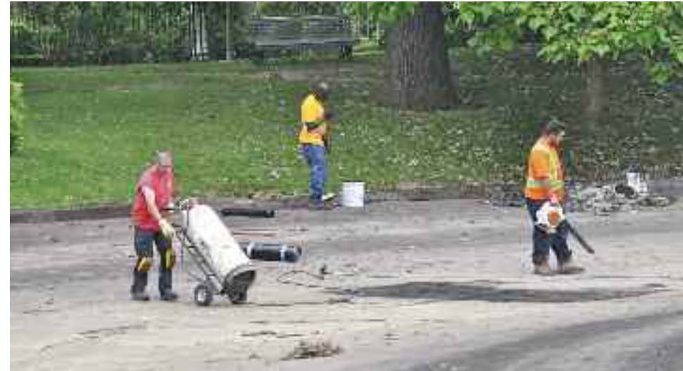
City workers were repairing damaged sections of the pond’s membrane in Westmount Park on July 4. Perhaps the work will repair the leak that is contributing to water issues at the arena/pool construction site (see July 2, p. 1).
