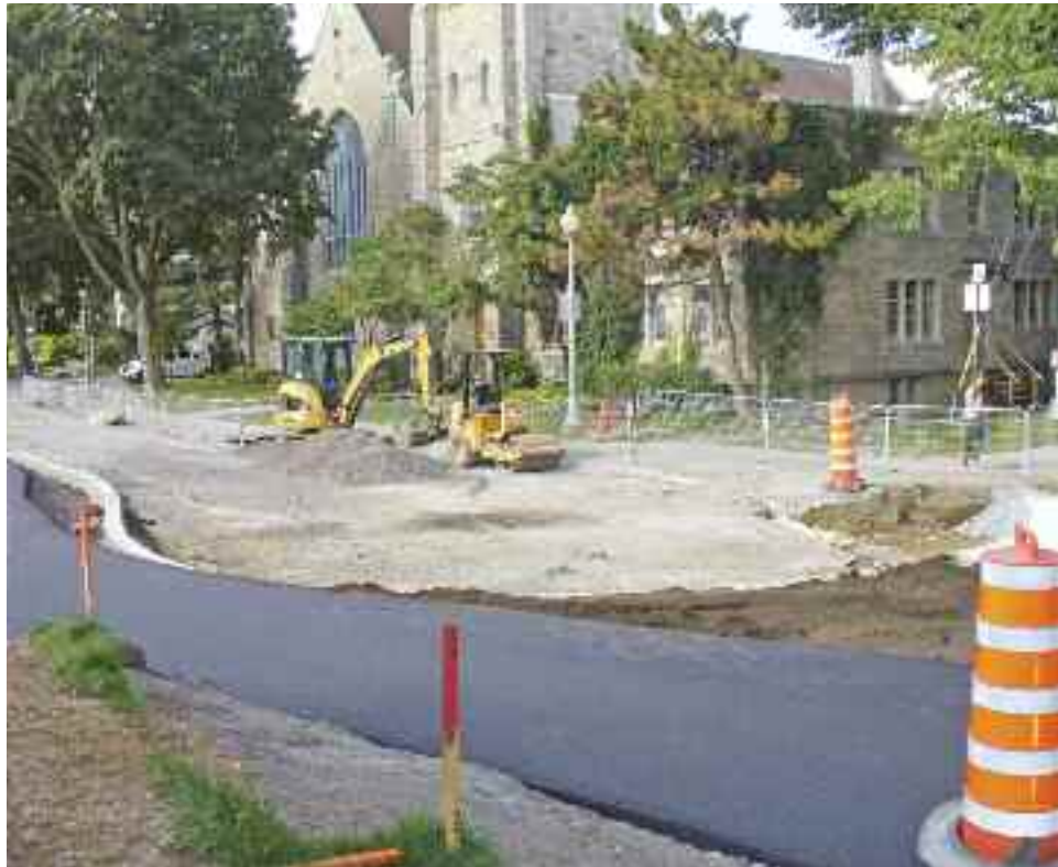
Work proceeds to complete the de Maisonneuve project in front of Westmount Park Church August 28.
