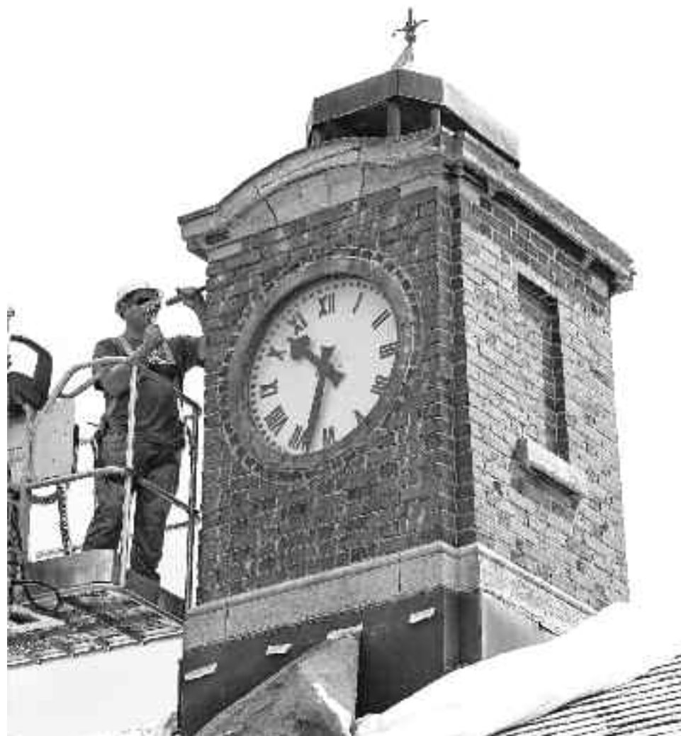
Pascal Rolland of Maçonnerie Denis Rolland does some restoration work to the brick facing of the clock tower building in King George (Murray) Park, facing Westmount Ave. August 19. The restoration project includes repairing the comfort station exterior as well. Photo: Robert J. Galbraith
