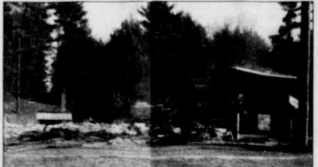
On March 25 the River View Inn (R.V.I.) in Norway Bay was torn down. The R.V.I. was originally built in 1908. In its place townhouses are going to be built.
