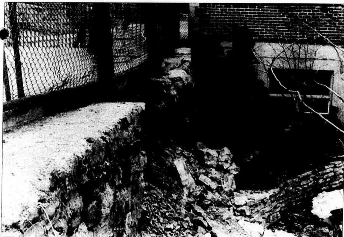
This collapsed retaining wall was scheduled for repairs by the public works department but it gave way before the tenders could go out. "It got to us before we could get to it," said Mayor Peter Trent.
