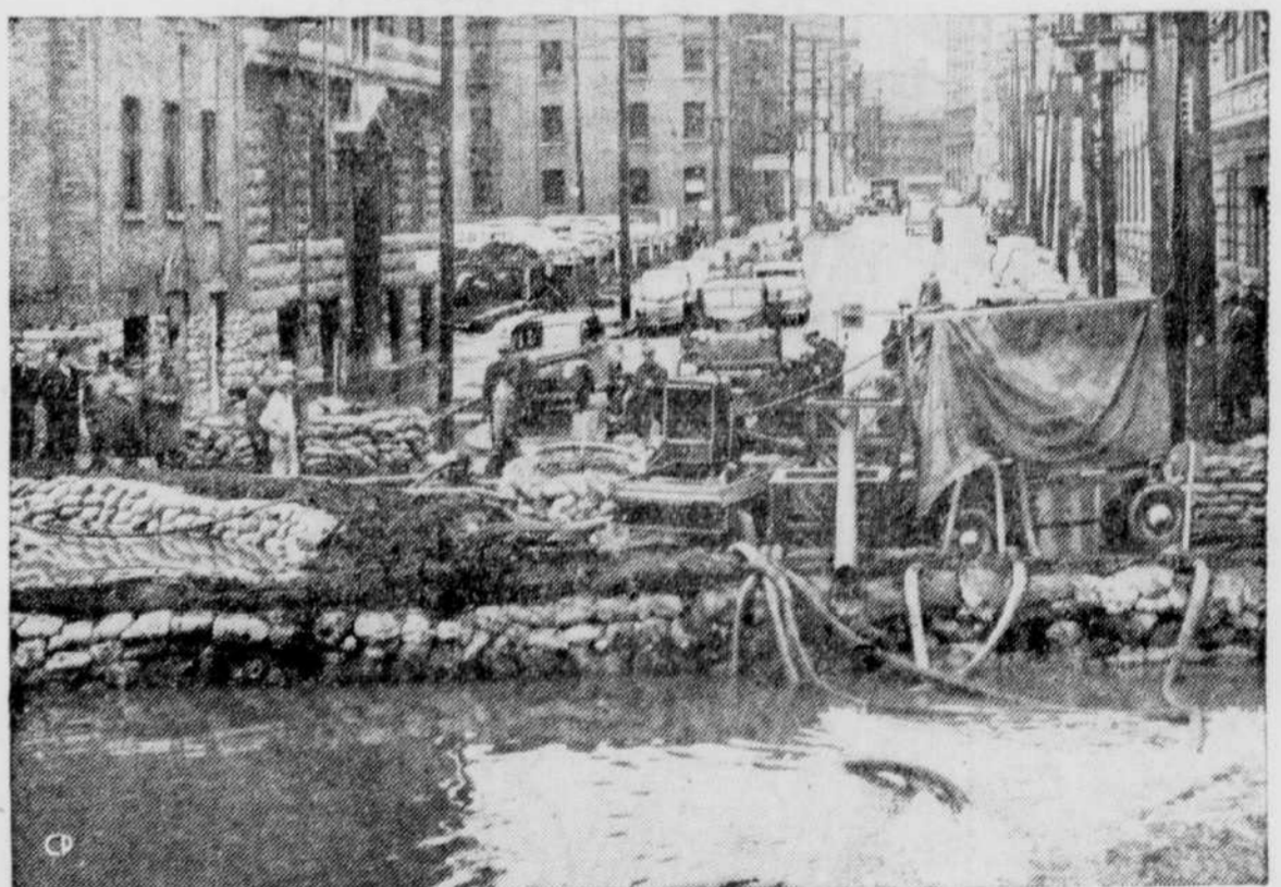
Red River flood waters fight to crack this rampart at the foot of Lombard street in downtown Winnipeg. Pumps shown in the foreground are drawing water from a backed-up sewer and tossing it over the barricade.
