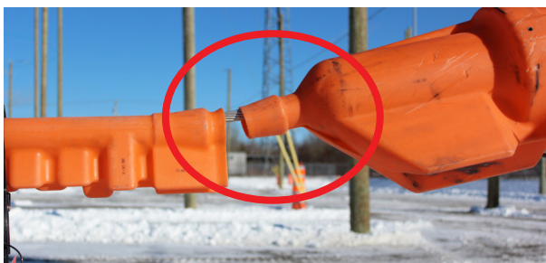
Part of conductor exposed due to faulty interlocking of conductor covers
