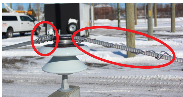
Loosened tie wires
