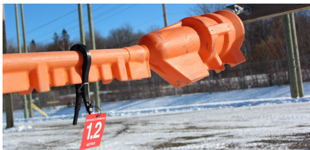
Correctly installed conductor covers
