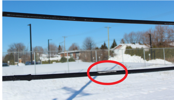
Damaged conductor sheath
