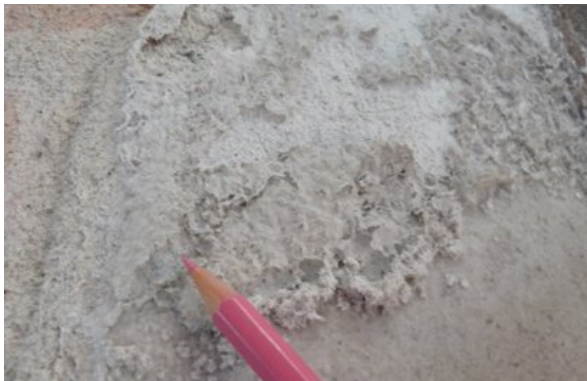
Figure 49 © Efflorescences salines ©CCQ/MCC, Elizabeth Cloutier 2013.
