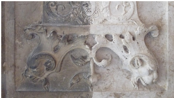
Figure 45 © Encrassement ©CCQ/MCC, Elizabeth Cloutier 2013.
